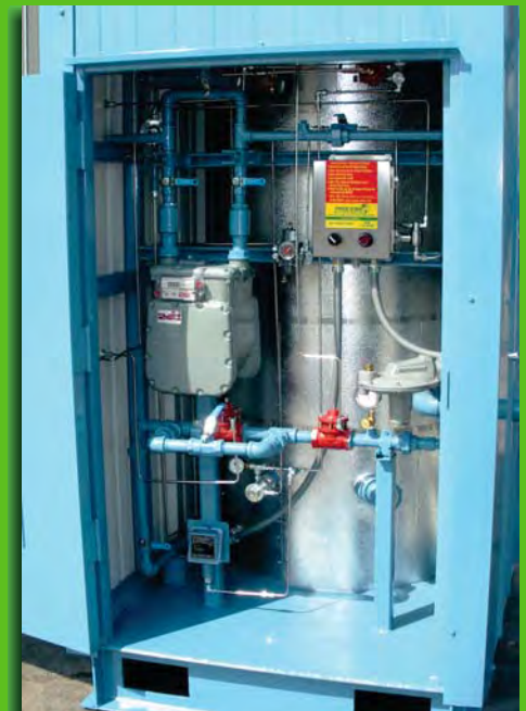
▲ Vertical Line Heater Interior
